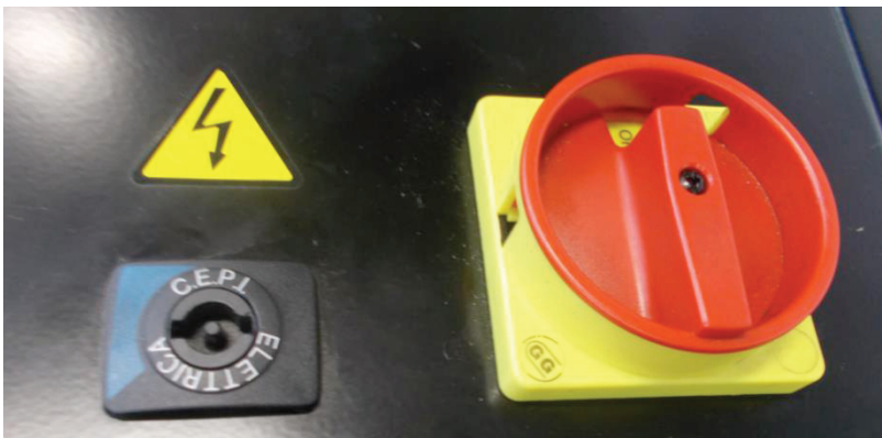
A: Electrical board
